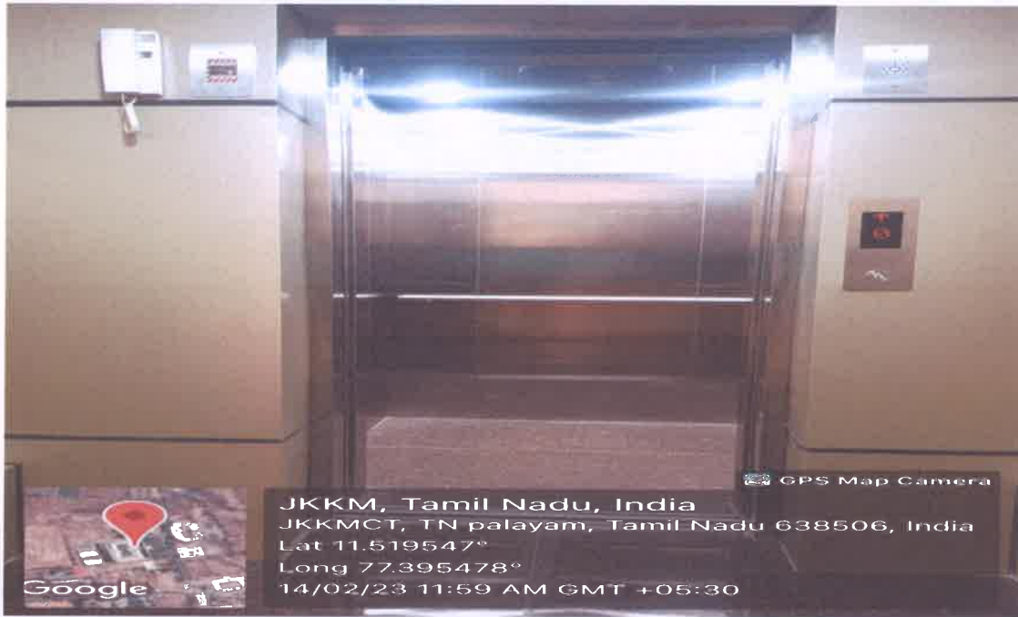
FIG 51: LIFT INSIDE VIEW
