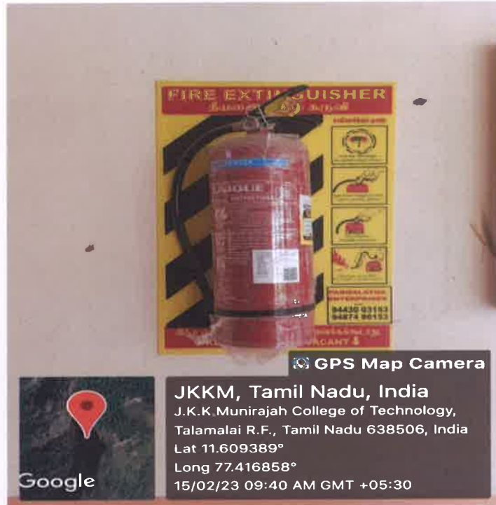
Photo of Fire Extinguisher
