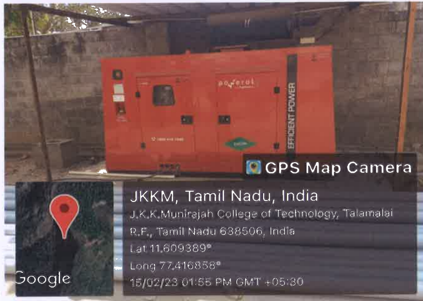
Photo of Generator
