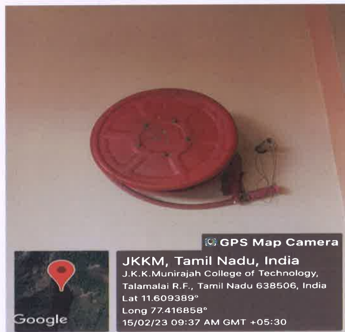
Photo of Fire Safety Pipeline
