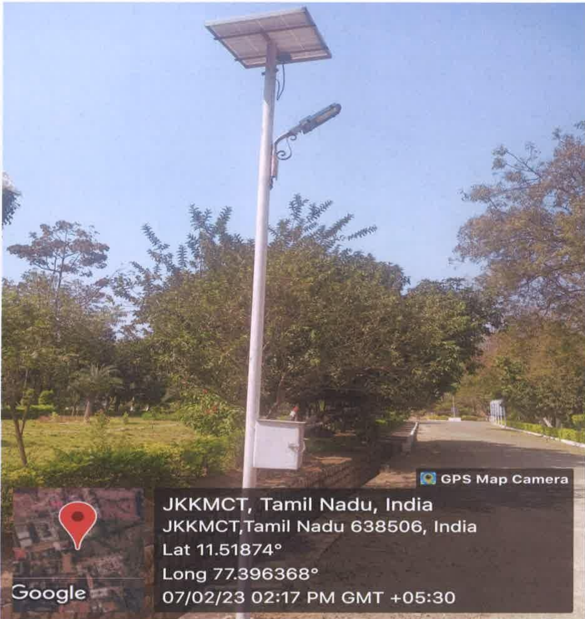
Photo of Solar Street Light in our college Main building
