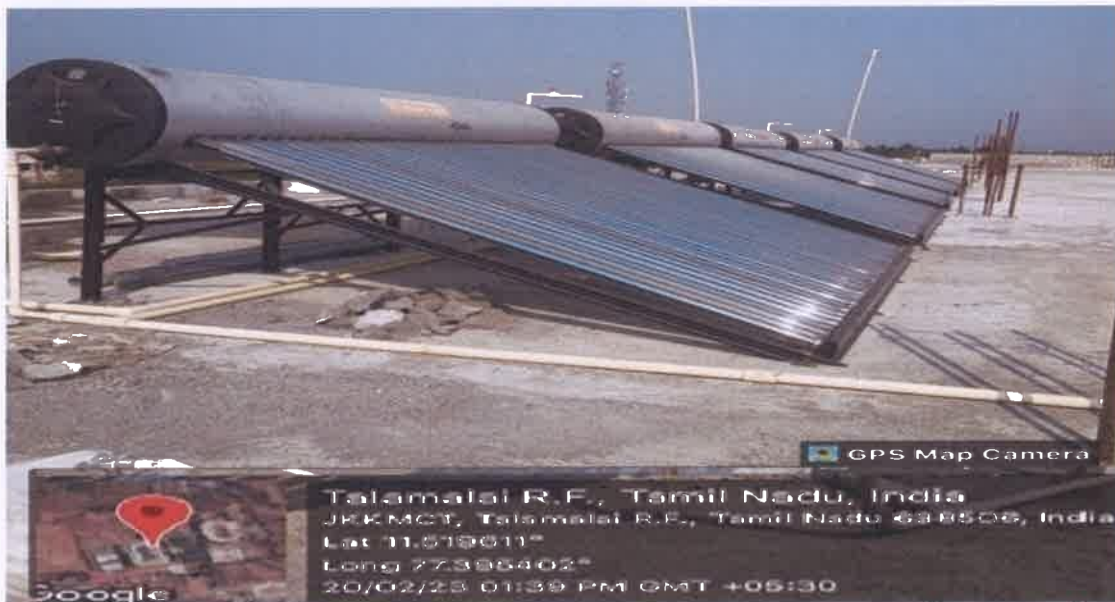
Photo of Solar Water Heater located at Girls Hostel
