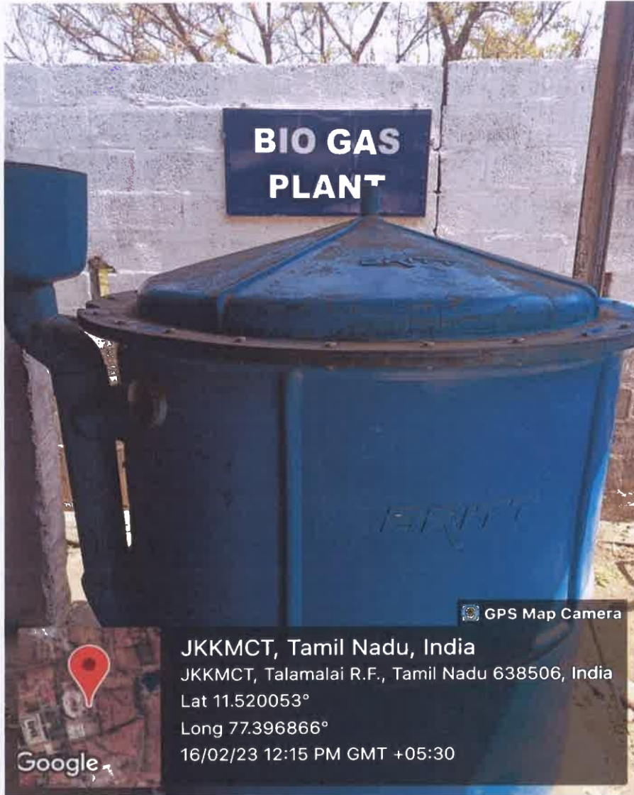
Photo of Biogas plant in our College Boys Hostel
