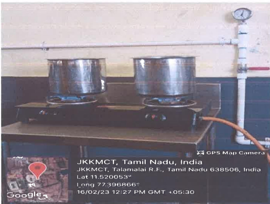
Photo of Unitization of Biogas in Pantry
