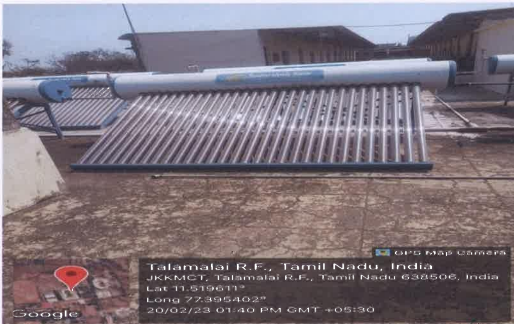
Photos of Solar Water Heater located at Girls Hostel
