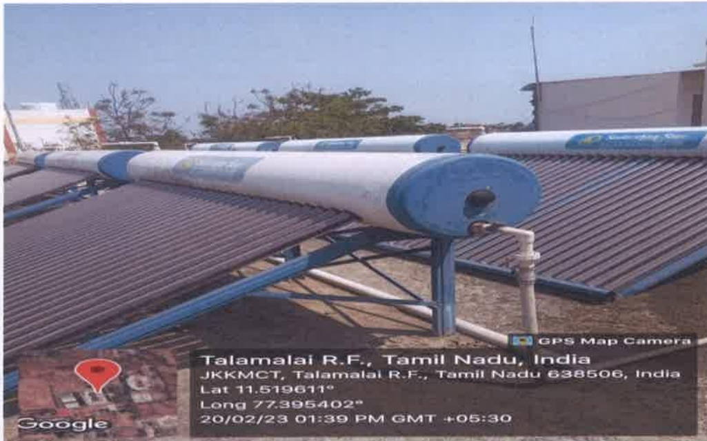
Photo of Solar Water Heater located at Girls Hostel
