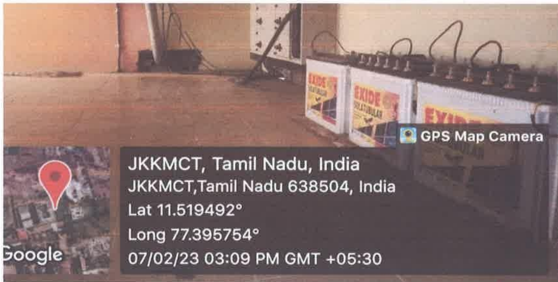
Photo of Solar Panel and Battery
