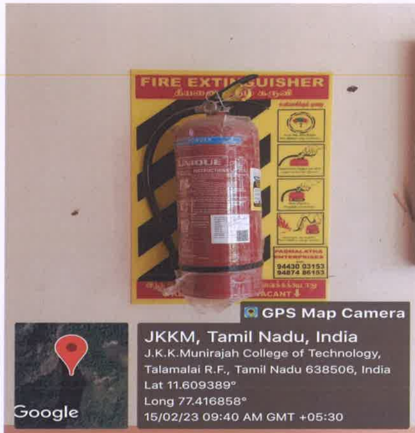
Photos of Fire Extinguishers
