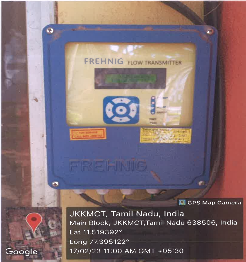
Photos of water meter in Main Block
