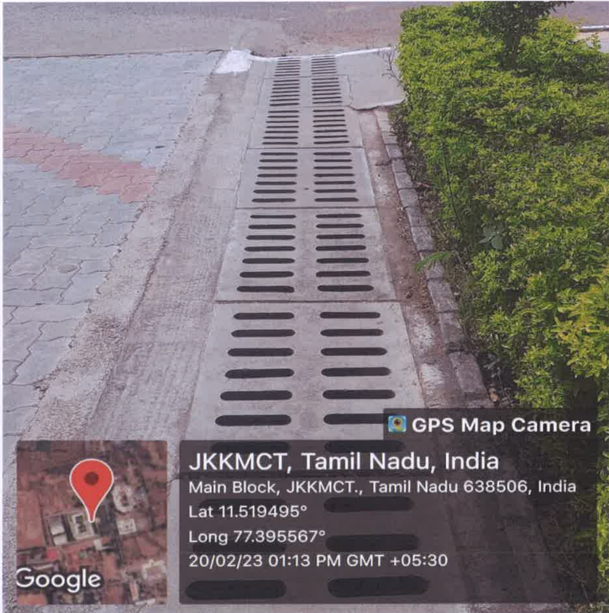
Photos of Distribution system in the campus
