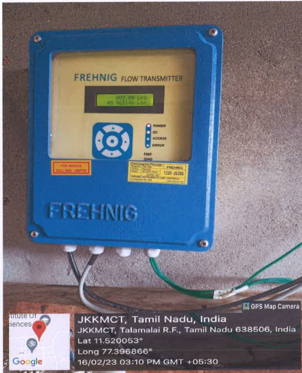
Photos of water meter in Boys Hostel
