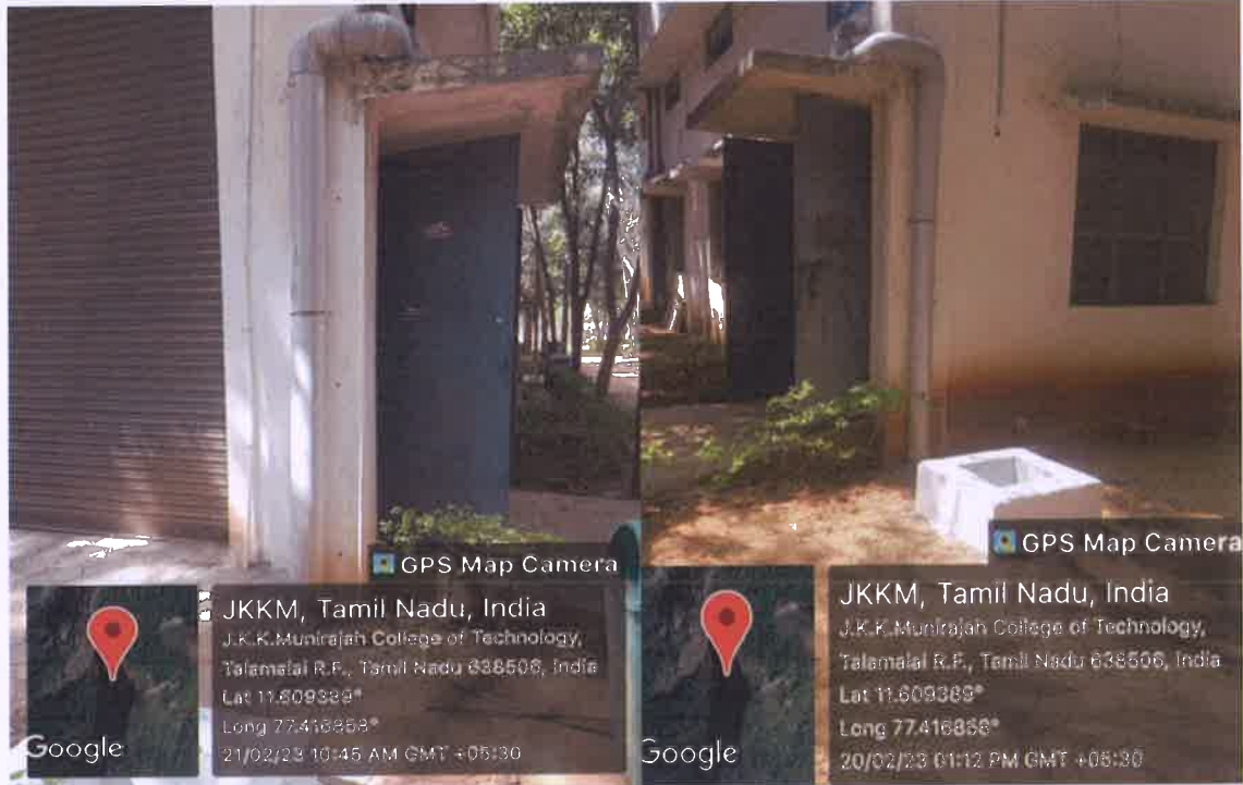
Photos of Rain water pipe lines in Laboratory
