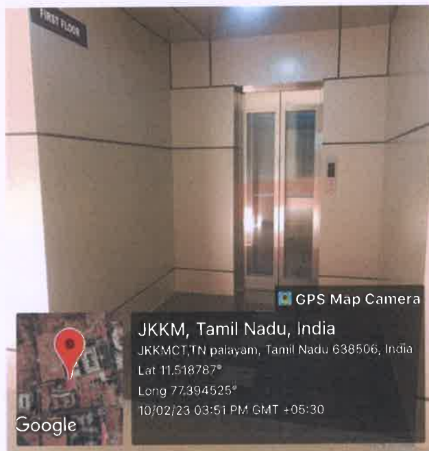
Photos of lift in the Ground, first, second & third floor
