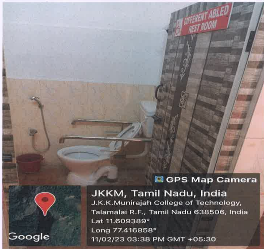
Photo for differently-abled washrooms
