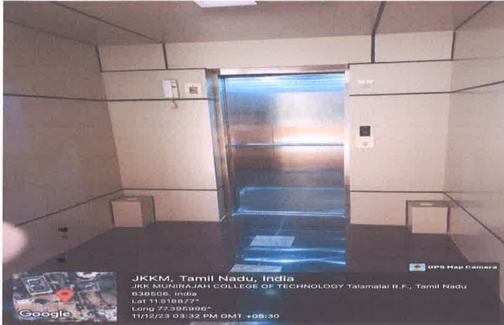
FIG 51: LIFT INSIDE VIEW
