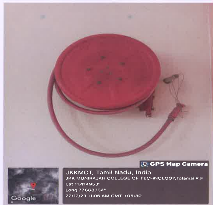
Photo of Fire Safety Pipeline
