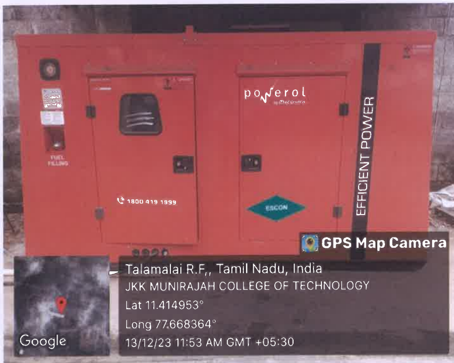
Photo of Generator
