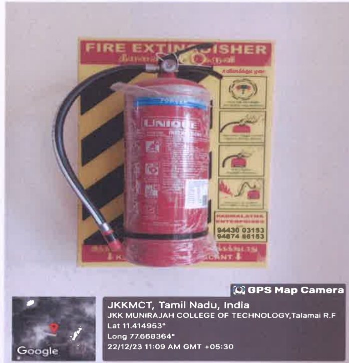
Photo of Fire Extinguisher
