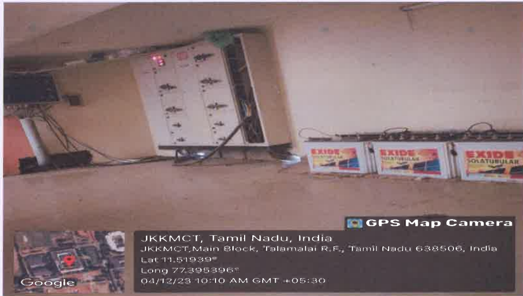
Photo of Solar Panel and Battery
