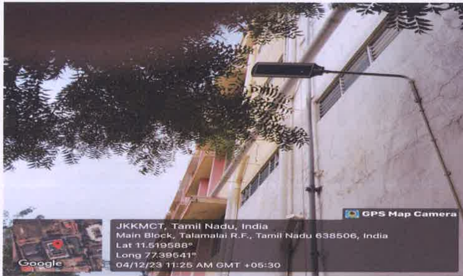
Photo of Sensor based automatic light located near Basketball ground
