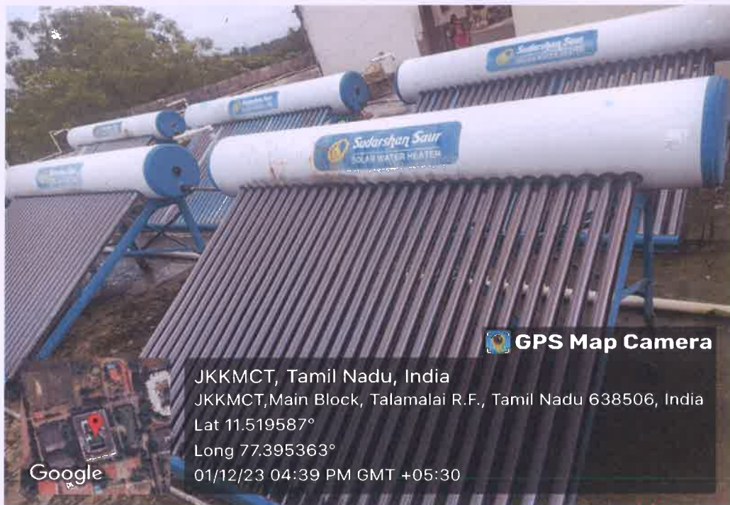
Photos of Solar Water Heater located at Girls Hostel
