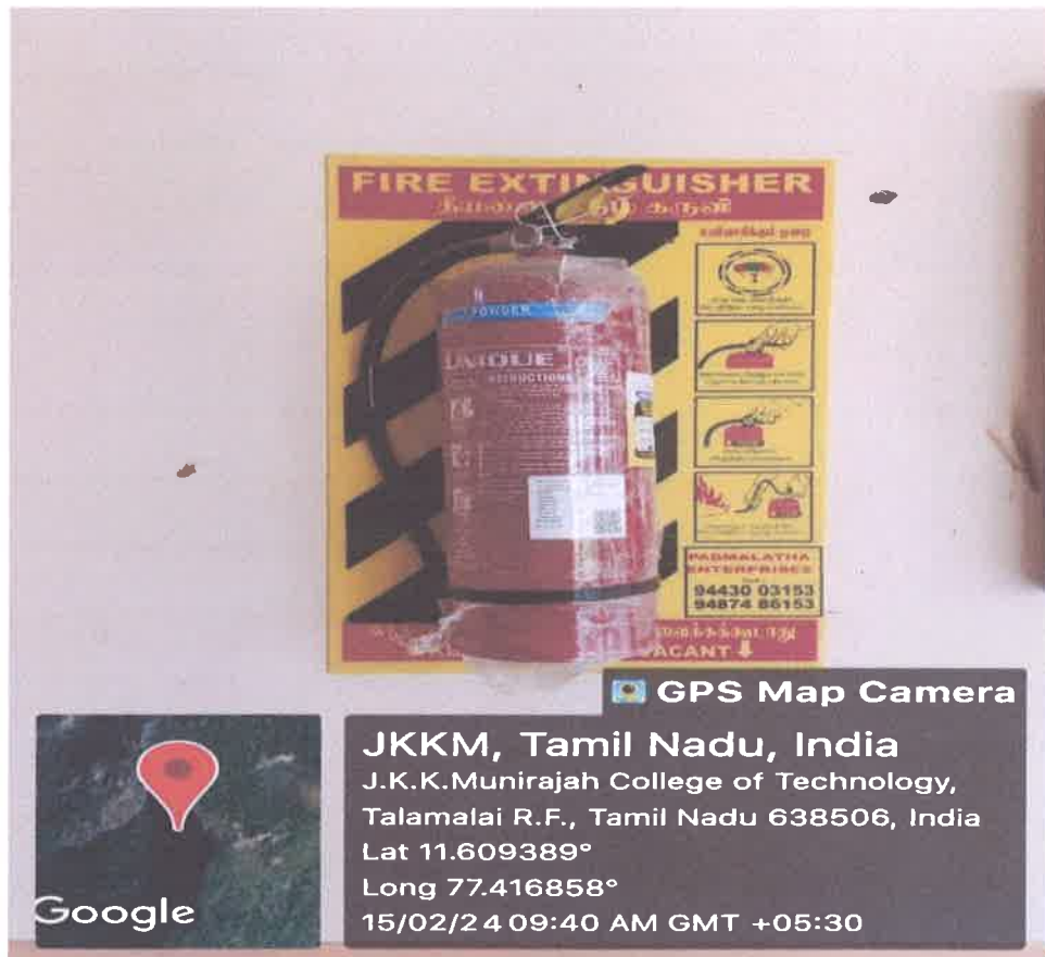
Photo of Fire Extinguisher
