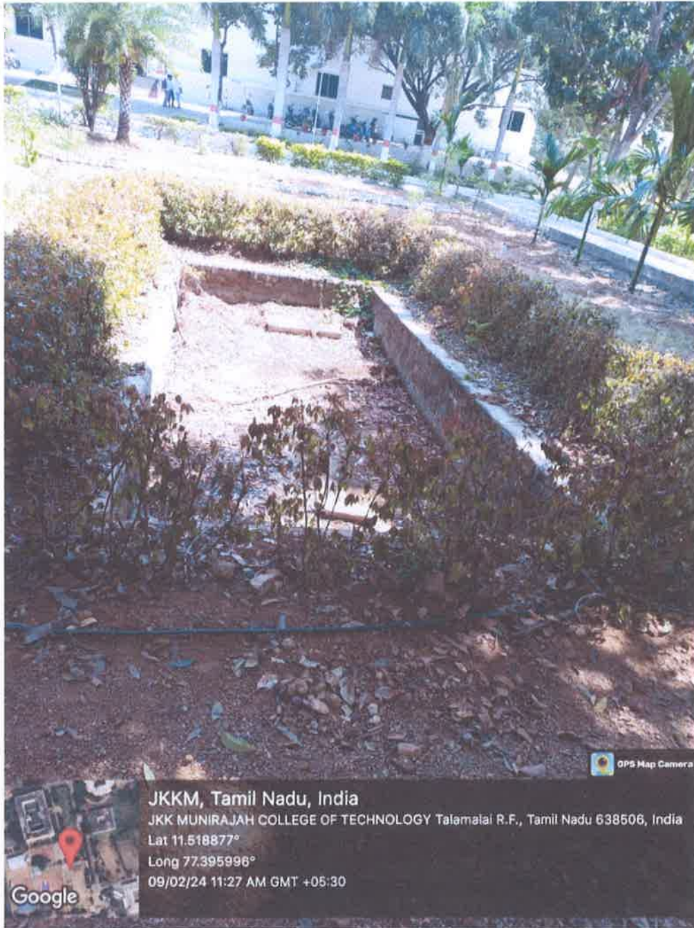
Photo of Septic tank located with our college backside
