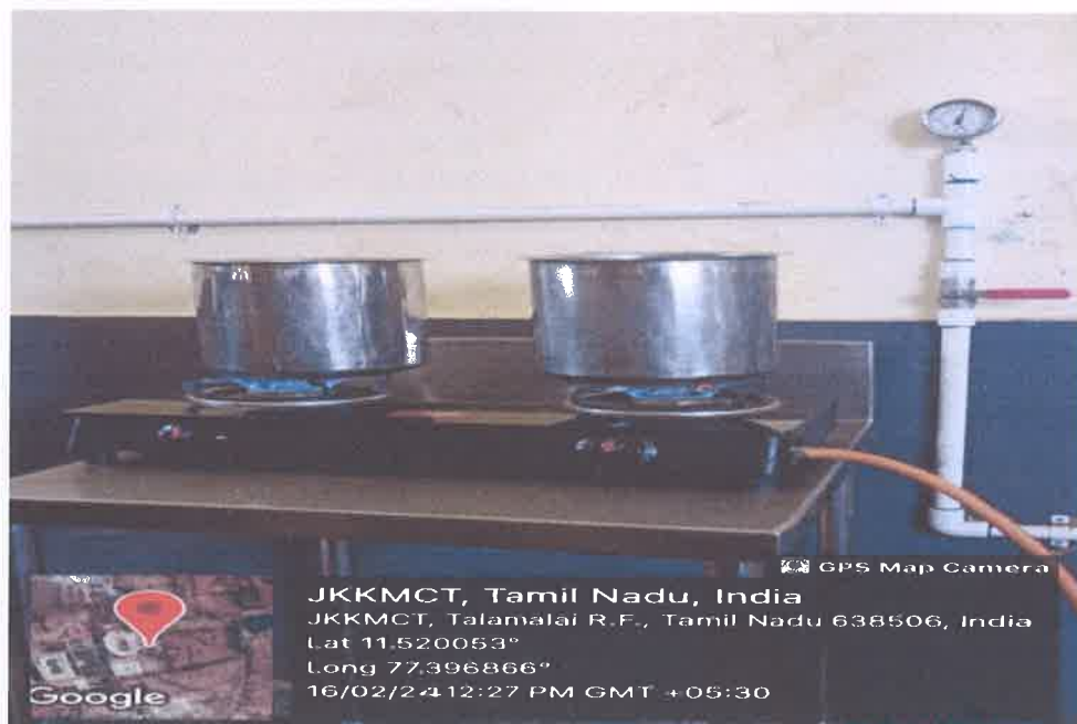
Photo of Unitization of Biogas in Pantry
