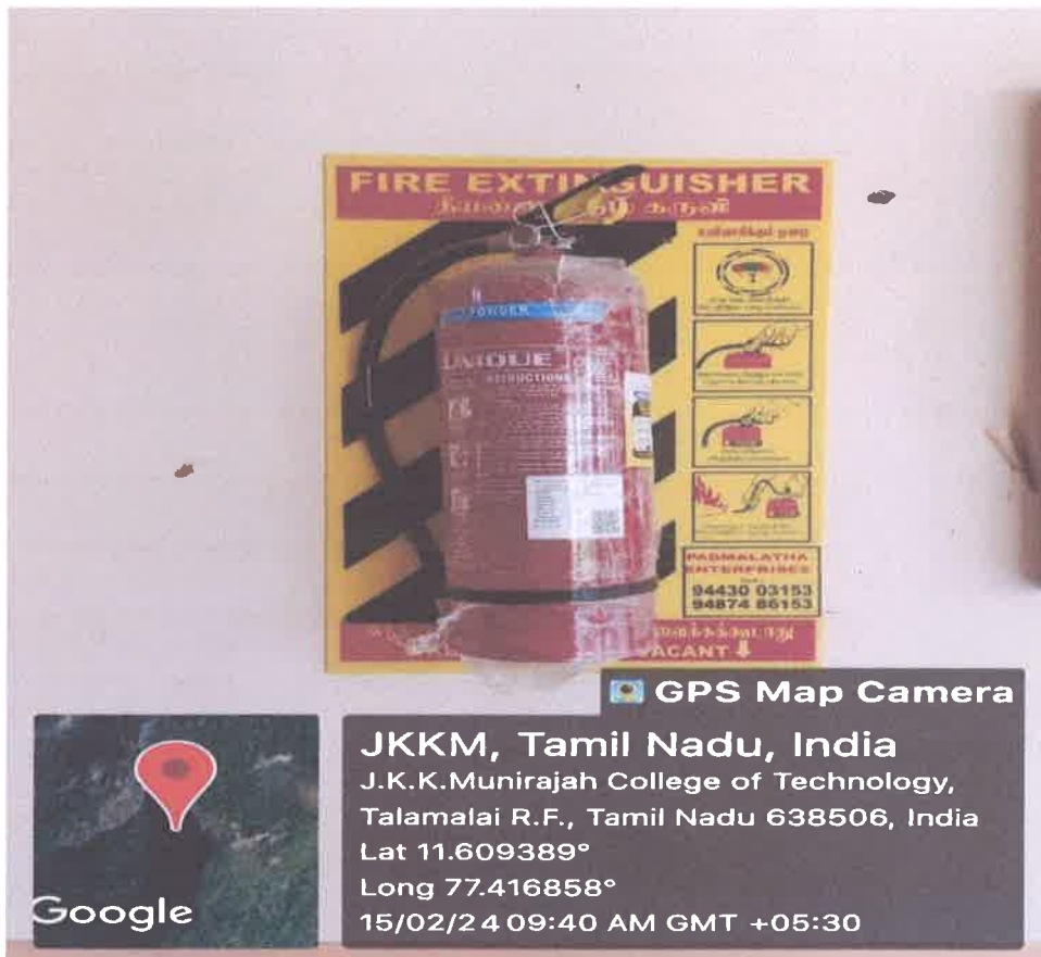
Photo of Fire Extinguisher
