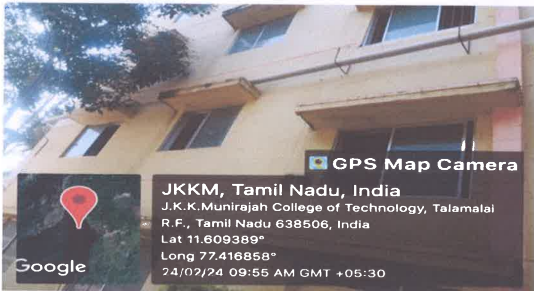
Photos of Rainwater pipe lines in Main Block backside
