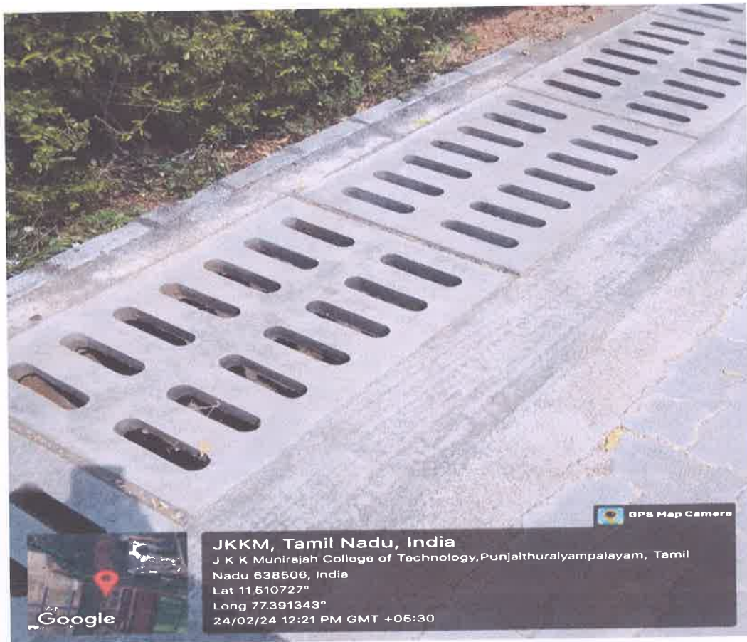
Photos of Distribution system in the campus
