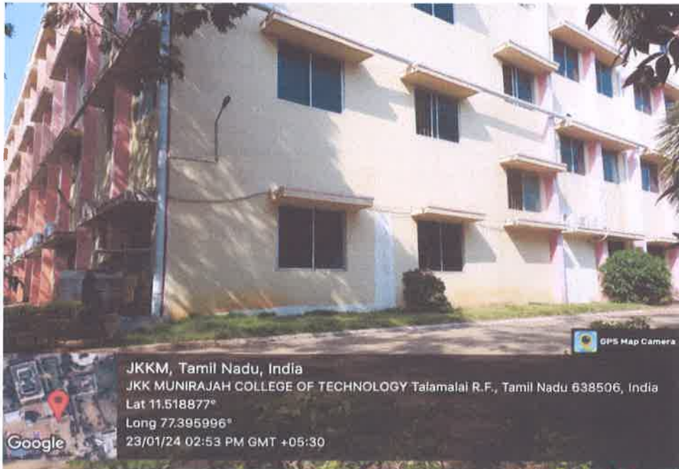
Photos of Rainwater pipe lines in Main Block
