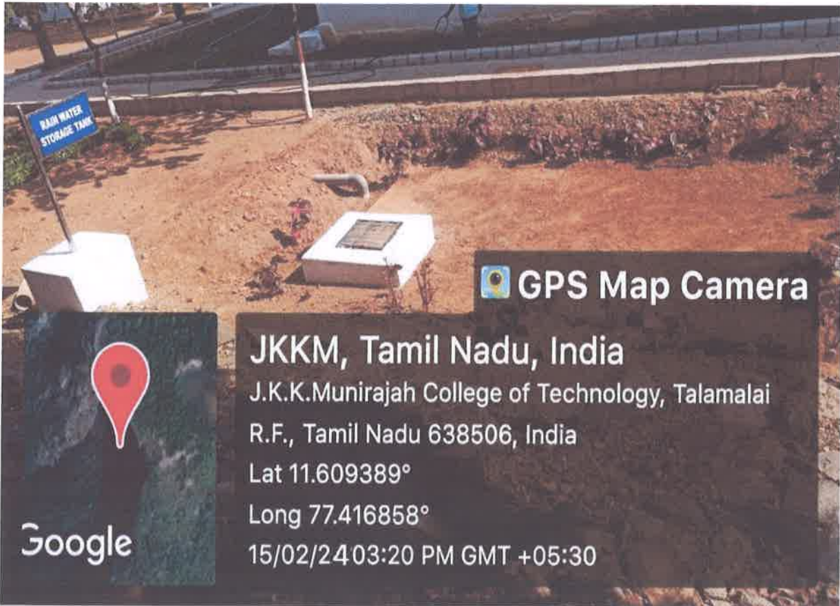
Photos of Rainwater storage tank
