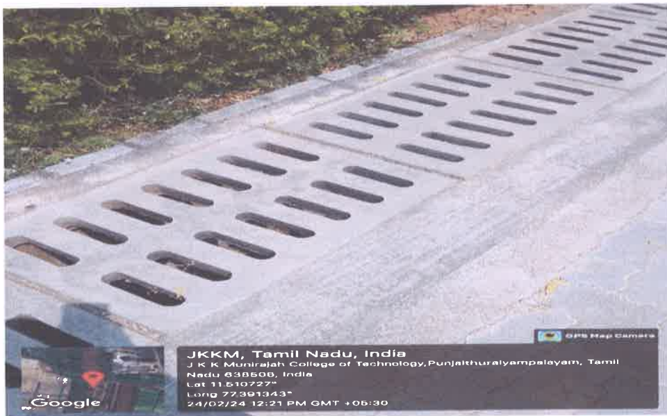
Photos of Distribution system in the campus
