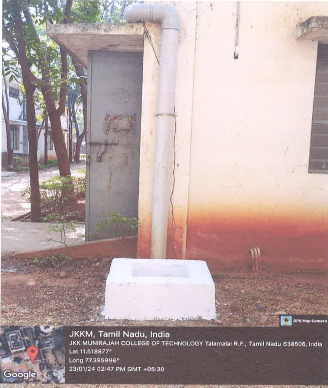
Photos of Rainwater pipe lines in Laboratory
