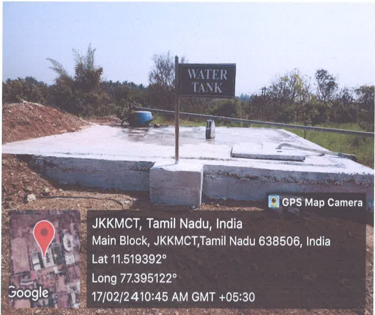
Photo of Water Tank in Boys Hostel
