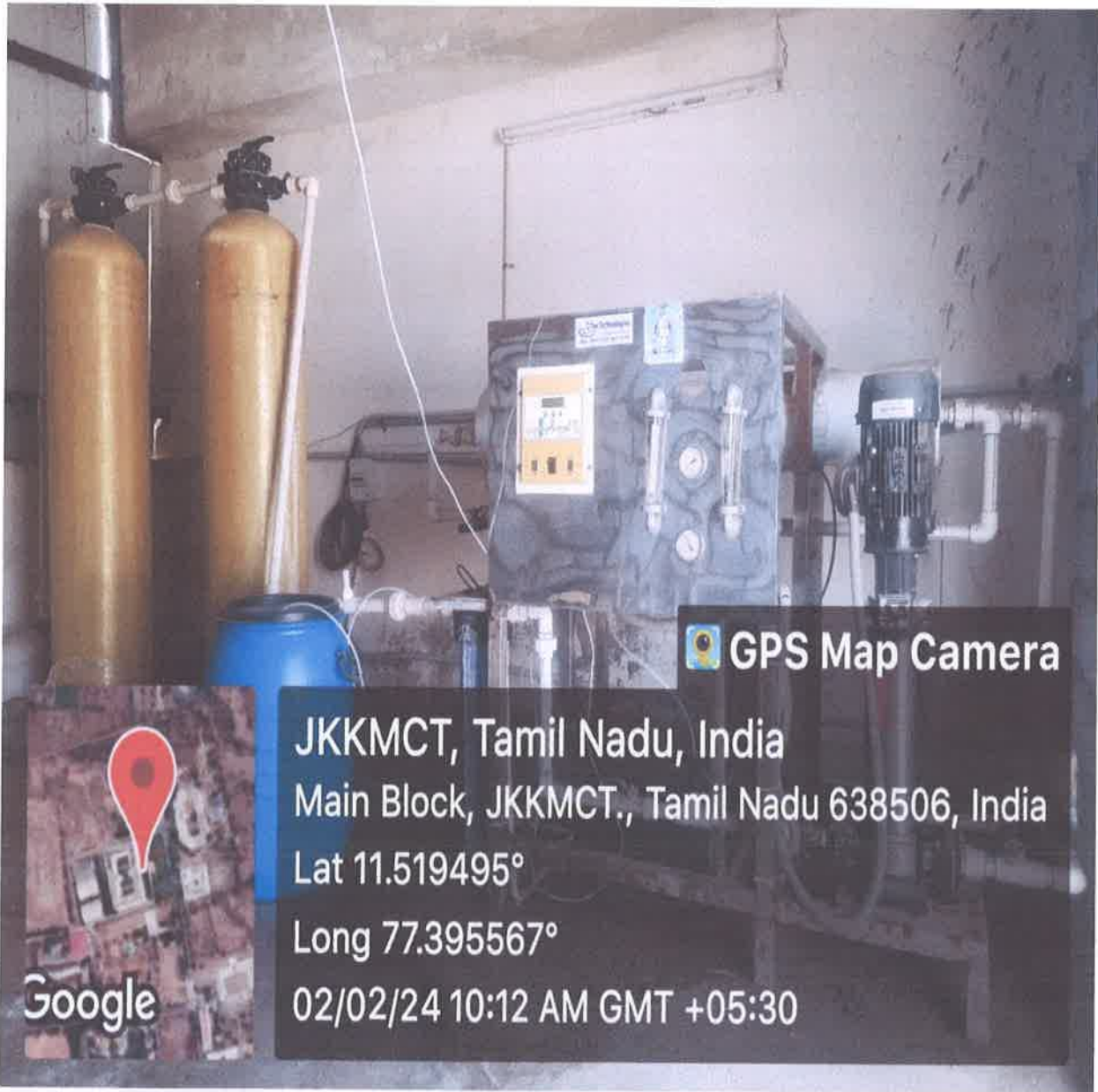
Photos of RO Water System College Main Block
