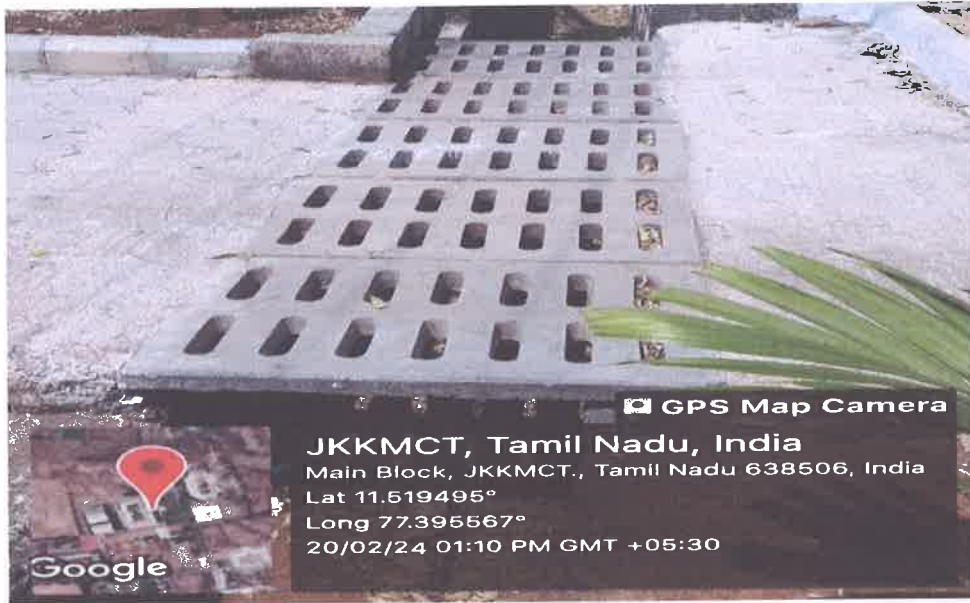
Photos of Distribution system in the campus
