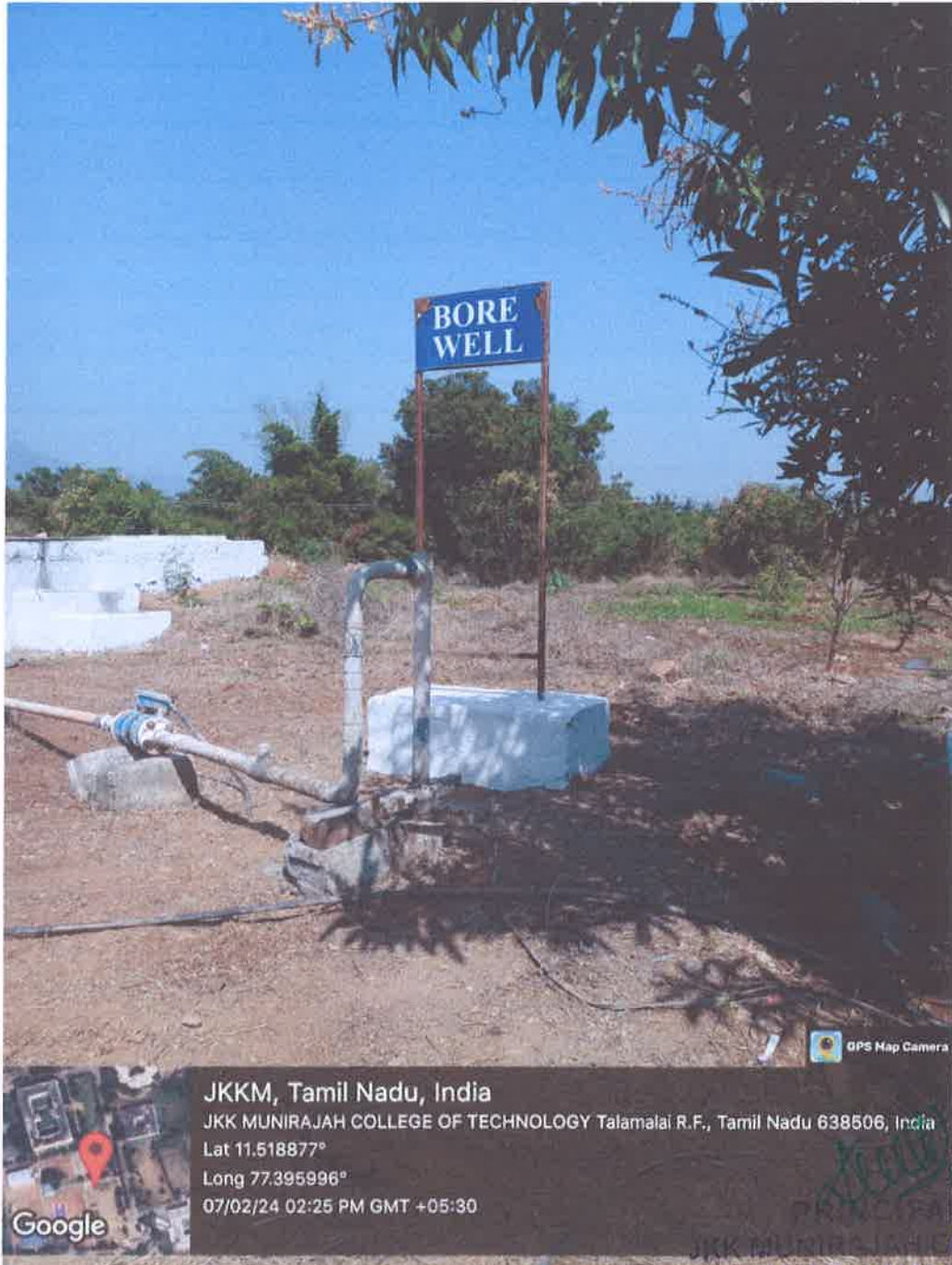
Photos of Bore Well in Rear Main Block
