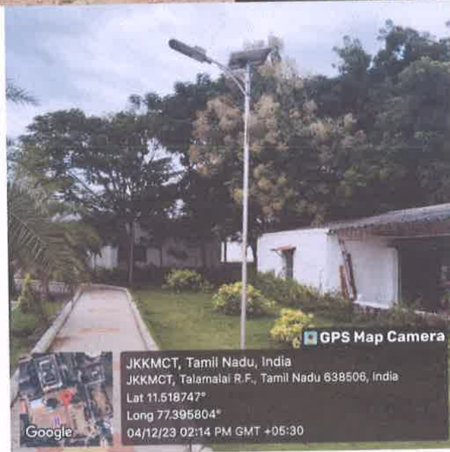
Photo of Solar Street Light in our college play ground
