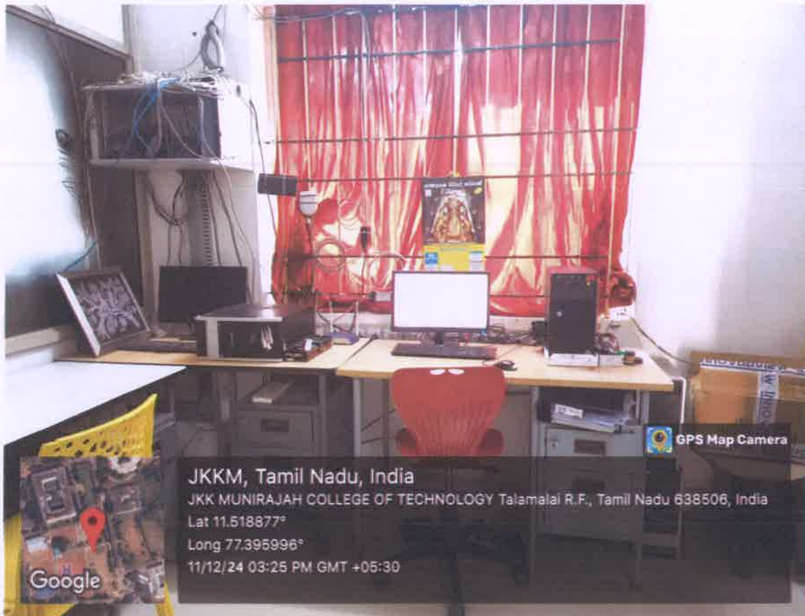
FIG 9 : SERVER ROOM INSIDE VIEW
