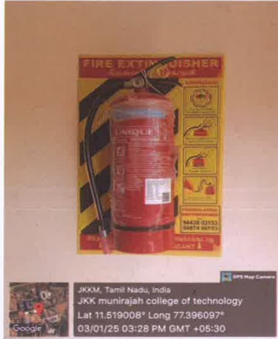
Photo of Fire Extinguisher
