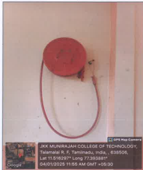
Photo of Fire Safety Pipeline
