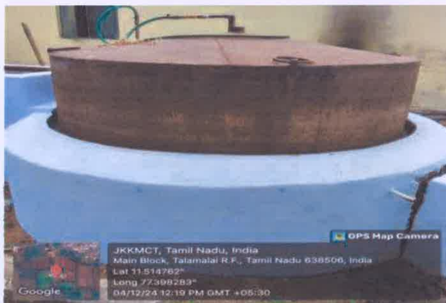
Photos of Biogas plant in our College Boys Hostel
