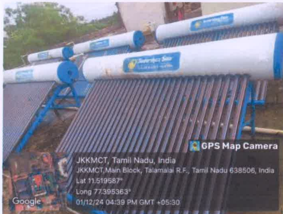
Photos of Solar Water Heater located at Girls Hostel
