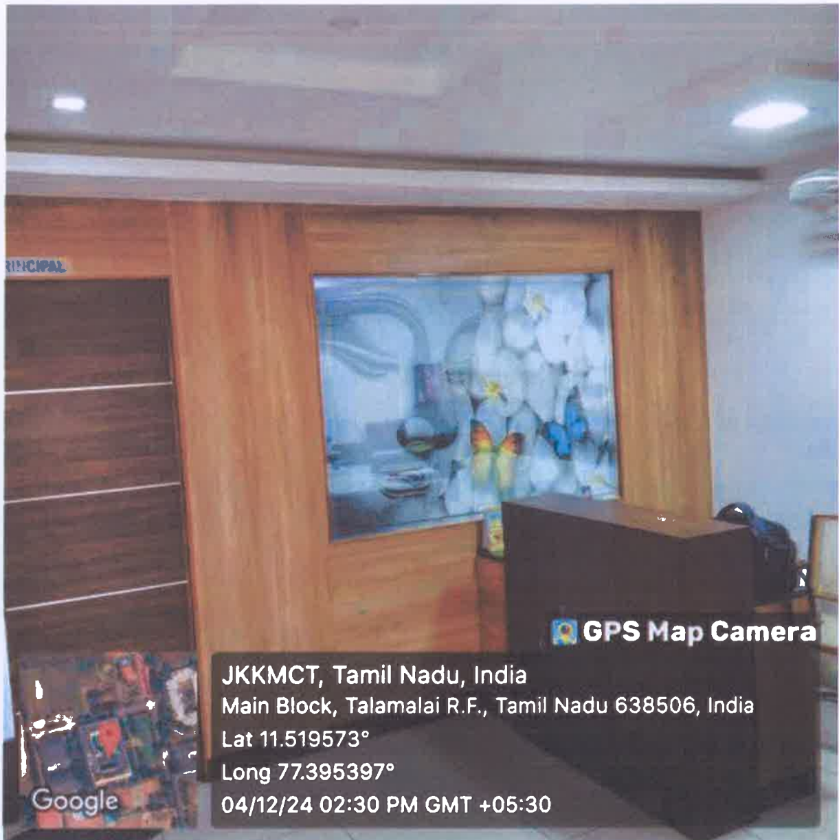
Photo of LED Bulbs in College office room
