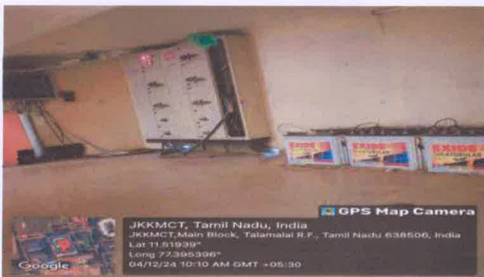
Photo of Solar Panel and Battery
