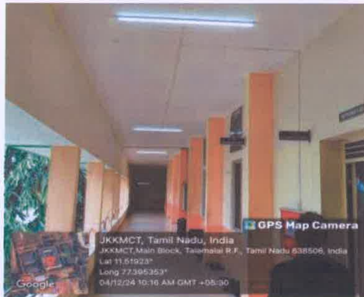
Photos of LED Bulbs in our College Main Building
