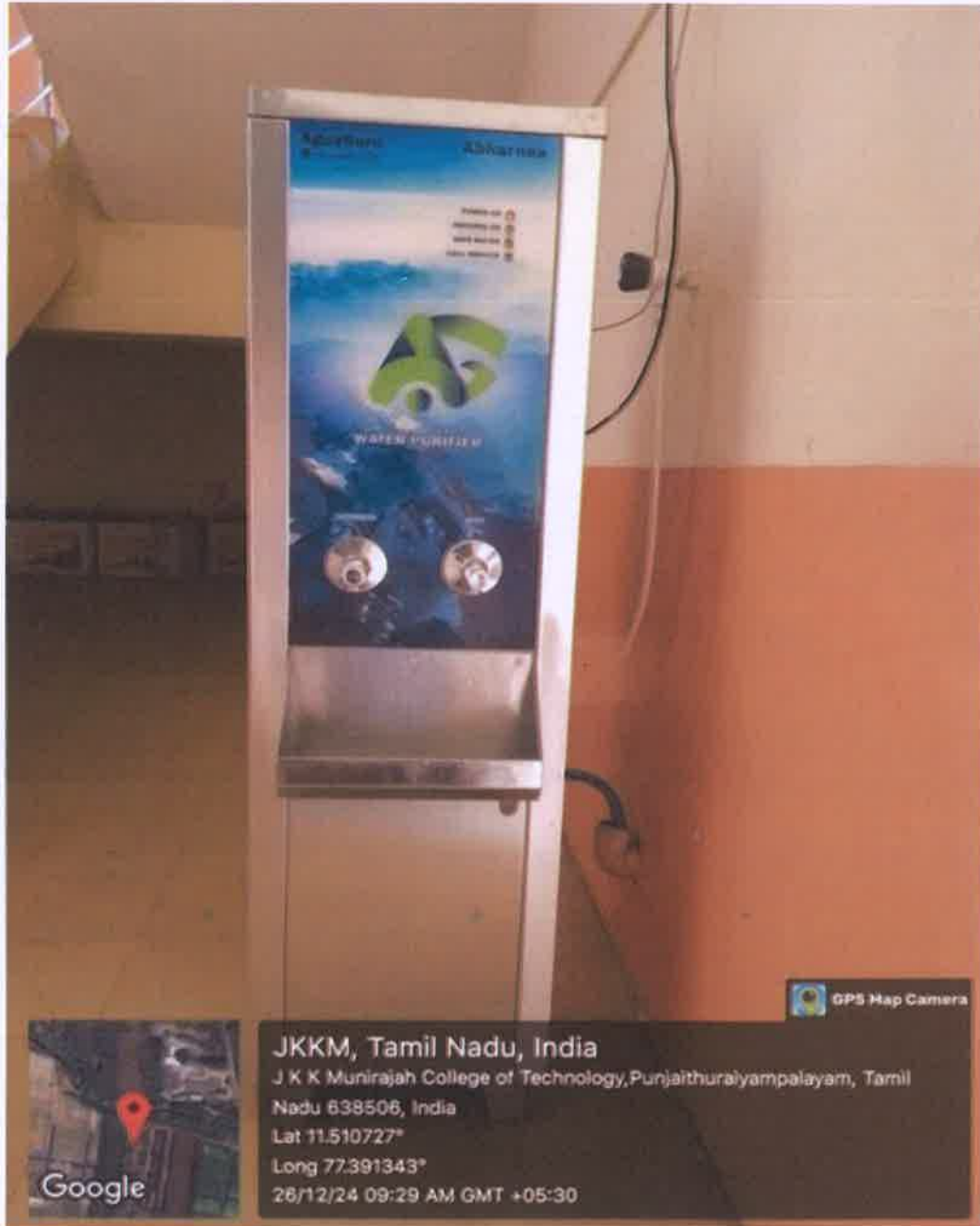
Photo of Liquid waste Management (Save Water)
