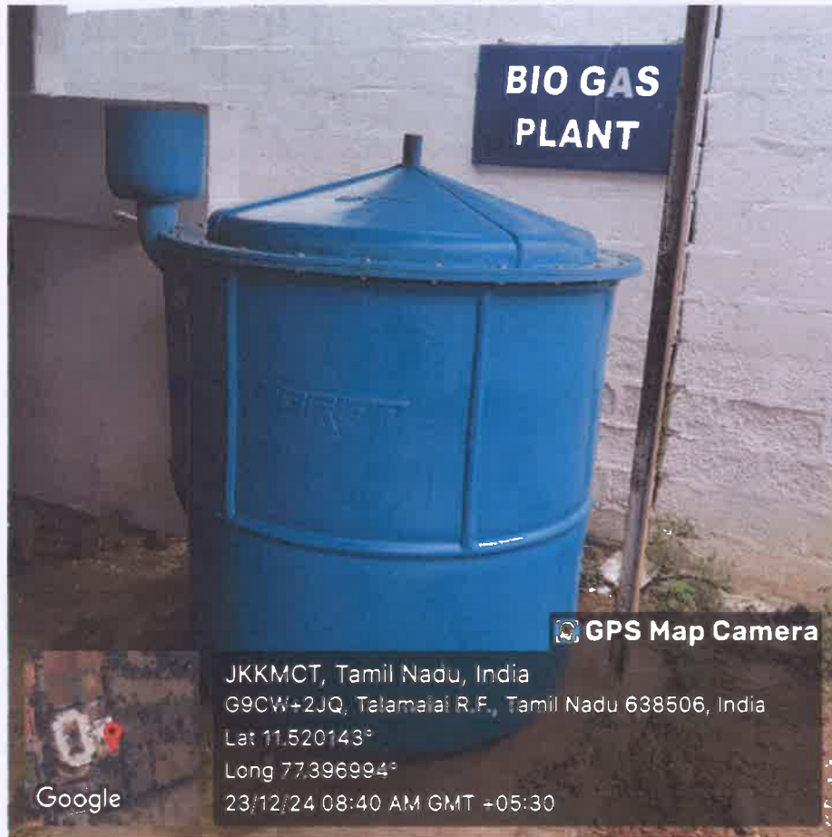
Photos of Biogas plant in our College Boys Hostel
