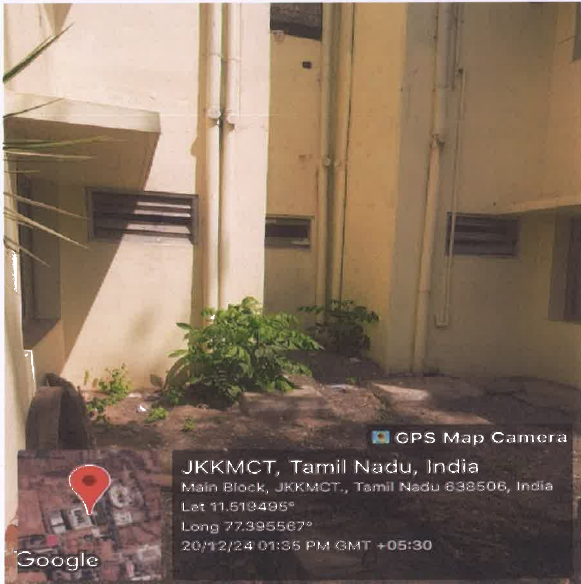
Photo of liquid waste Management pipe lines
