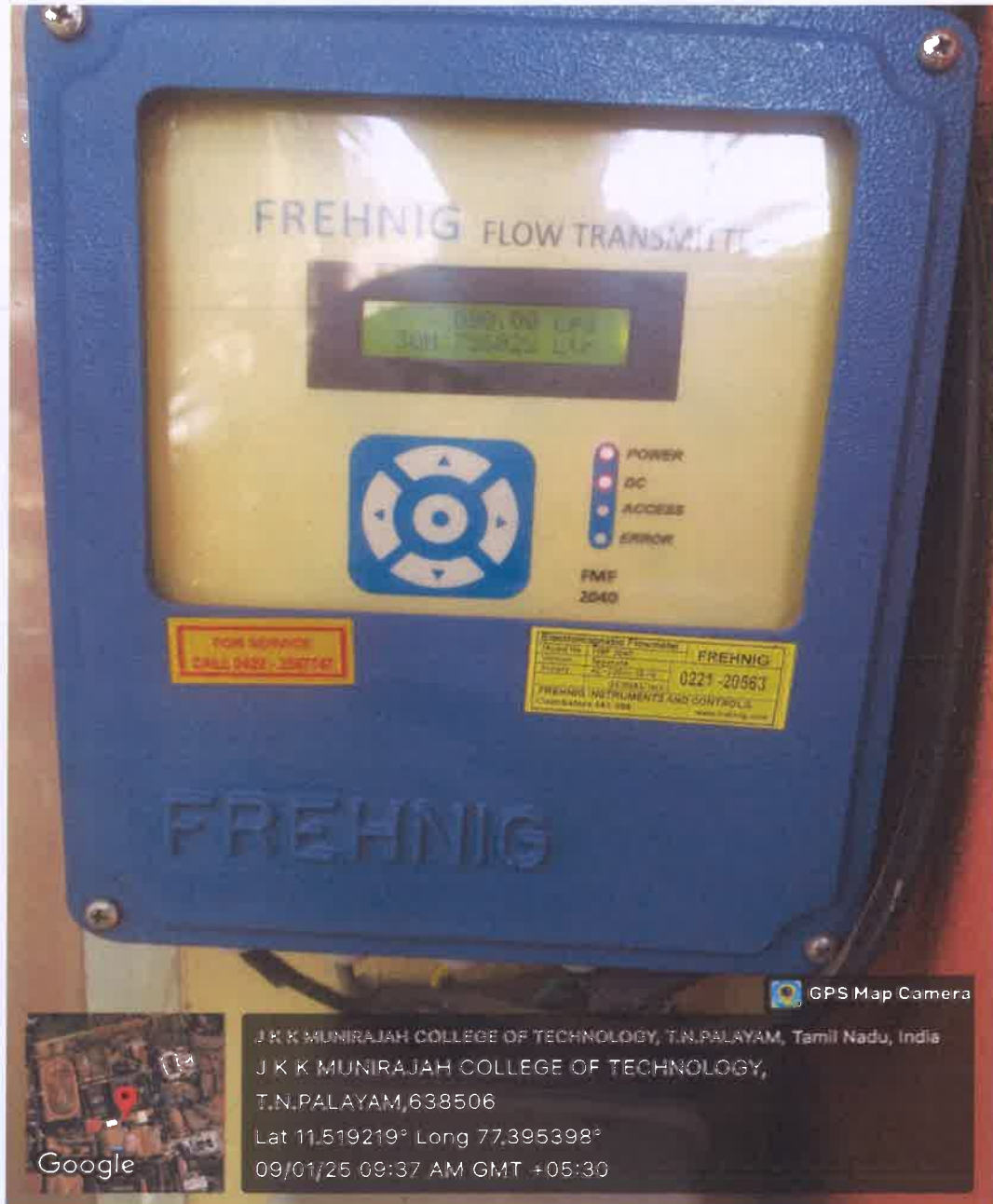
Photo of water meter in Boys Hostel
