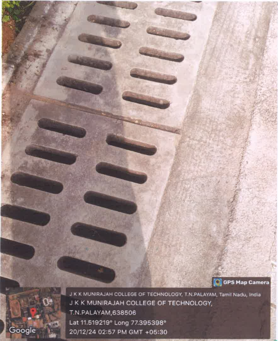
Photo of Distribution system in the campus
