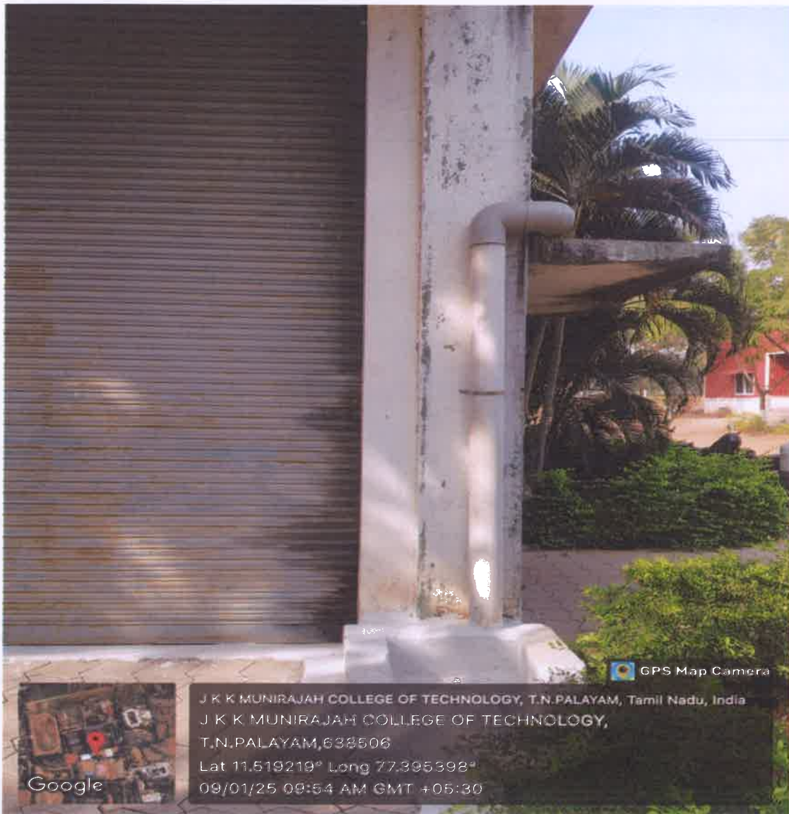
Photo of Rainwater pipe lines
