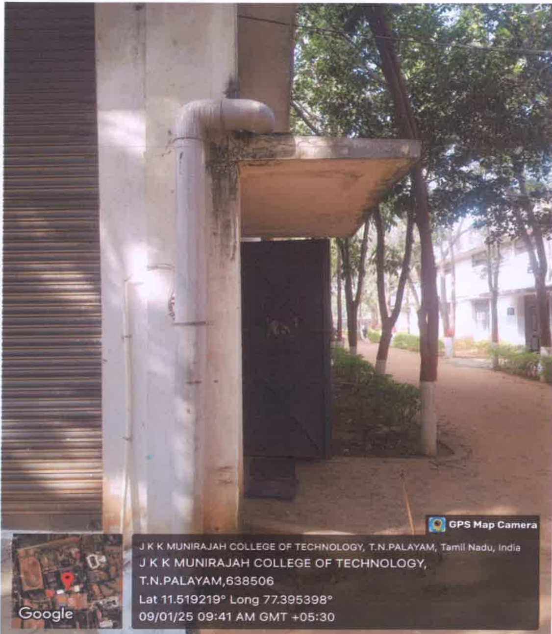
Photo of Rainwater pipe lines in Laboratory
