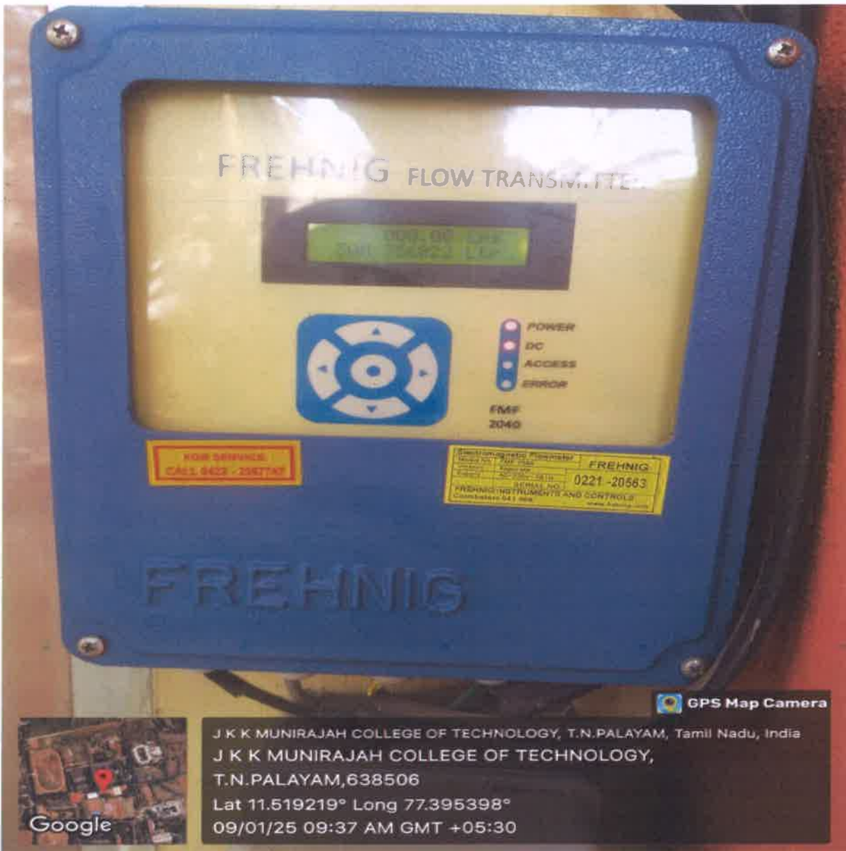
Photo of water meter in Rear Main Block
