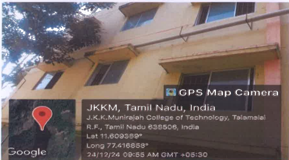
Photo of Rainwater pipe lines in Main Block backside
