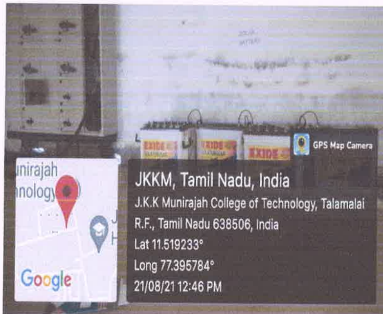
Solar Battery Located at Our College Main Building Ground Floor
