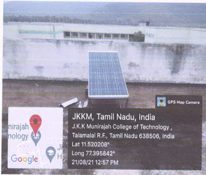
Solar Panel Located at Our Main Building Roof-Top
