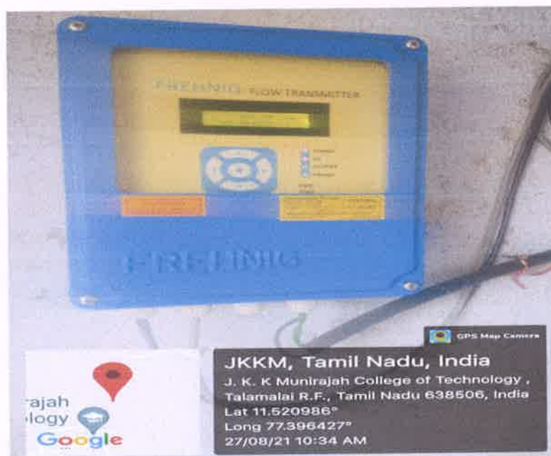
Water Meter fixed with Bore well
