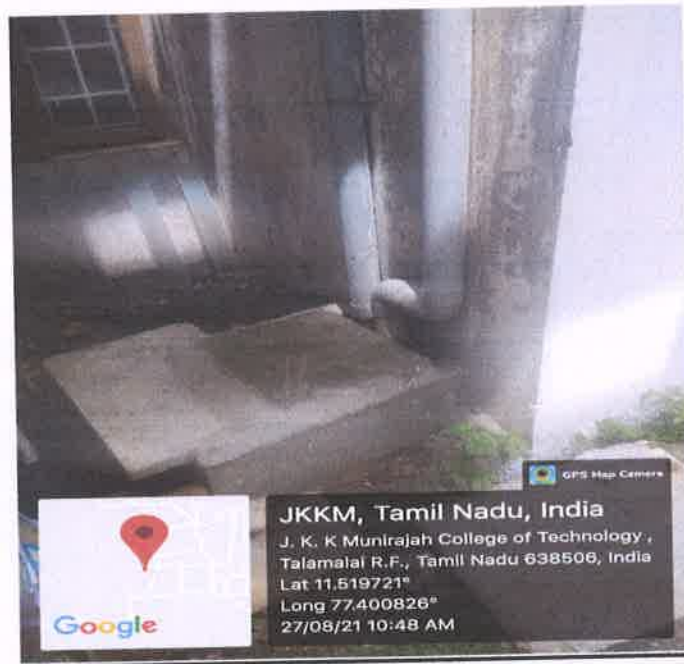
Rain water harvesting Camper in Main Building
