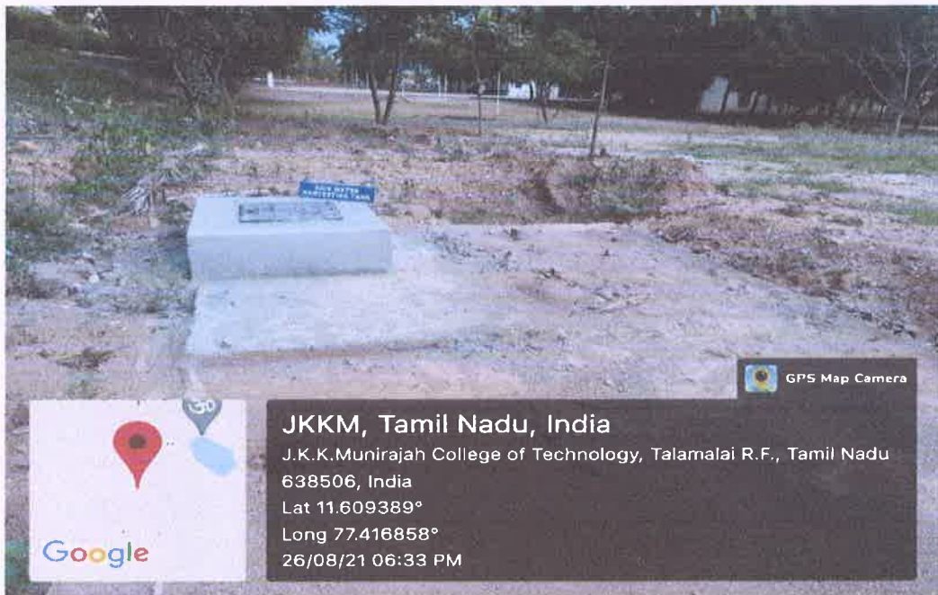
Rain Water Harvesting Tank located in below the Soak Pit
